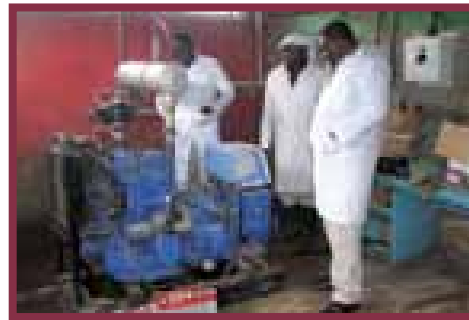
Biogas is converted into electricity
