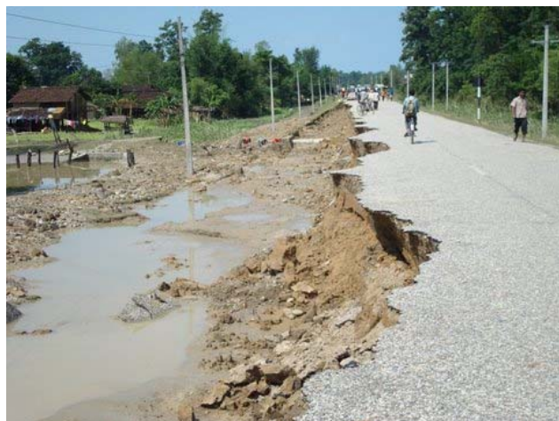
Intensity of road damage in Kanchanpur Photo source: UN OCHA
