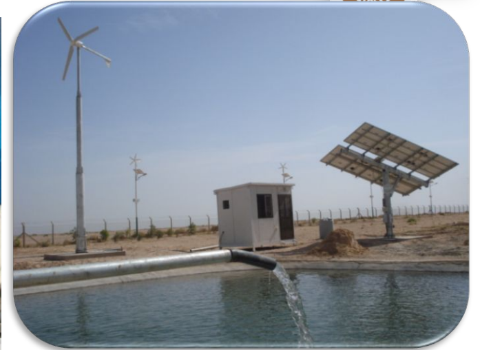
Renewable energy system
