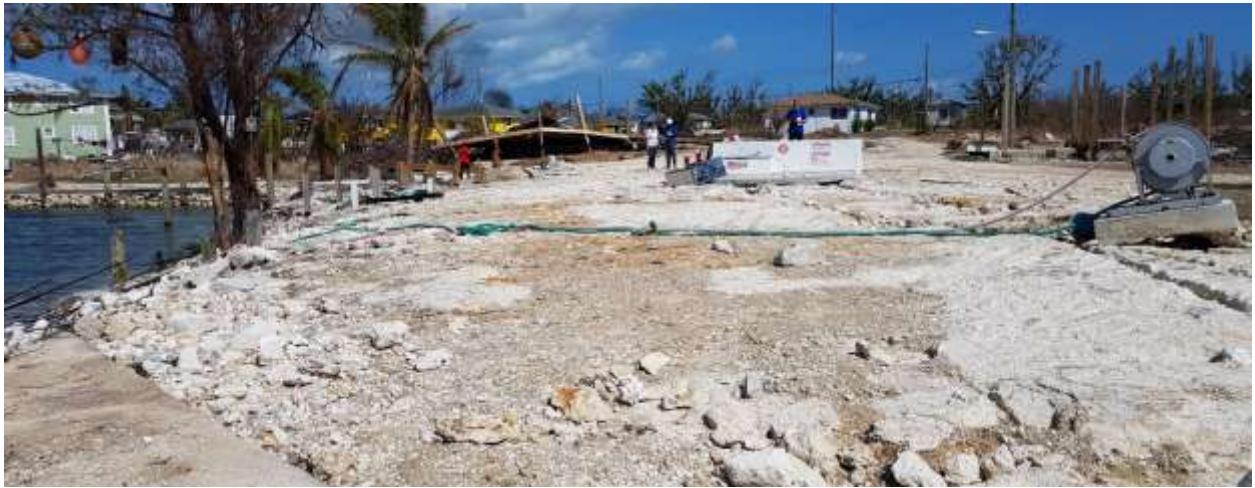
Figure 10. Damaged quay in Crown Haven (authors).
