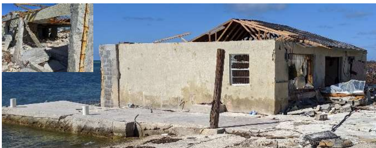
Figure 7. Destroyed buying station with concrete dock, in Mclean's Town. The dock is still usable, but the gas pump, which was standing next to the house wall, is gone. The small picture in the upper left corner shows the buying station from the dock side (authors).
