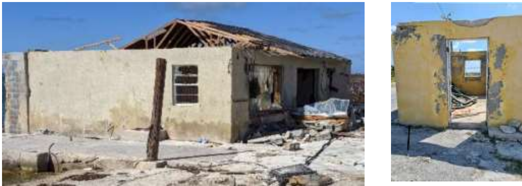
Figure 1 – Buying station buildings (pictures taken after Hurricane Dorian)
