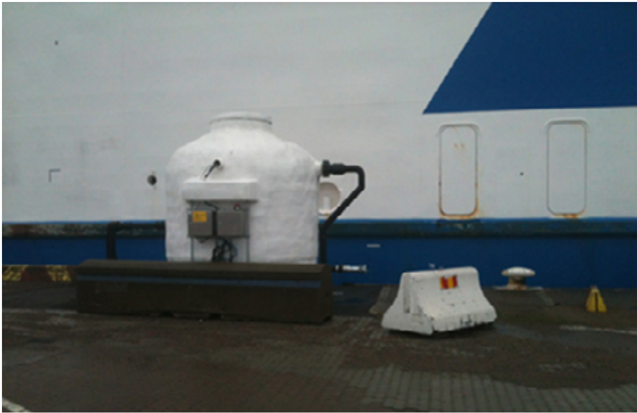
Figure 9: Sewage collection in port of Trelleborg, Sweden (Photo credit: Clean Baltic Sea Shipping)
