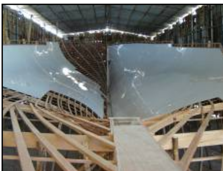
One off mould for 30 m pole- and line boat under construction in Viligili village
