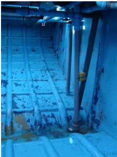
Baitwell. Plugs for watercirculation towards side. Split plastic pipes used as mould for stiffeners.
