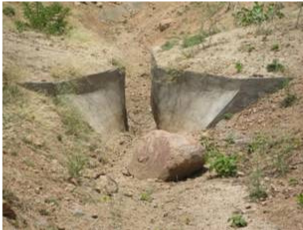
Plate 6. Secondary canal equipped with a flume in ALBC, no gauge installed and presence of rocks .
