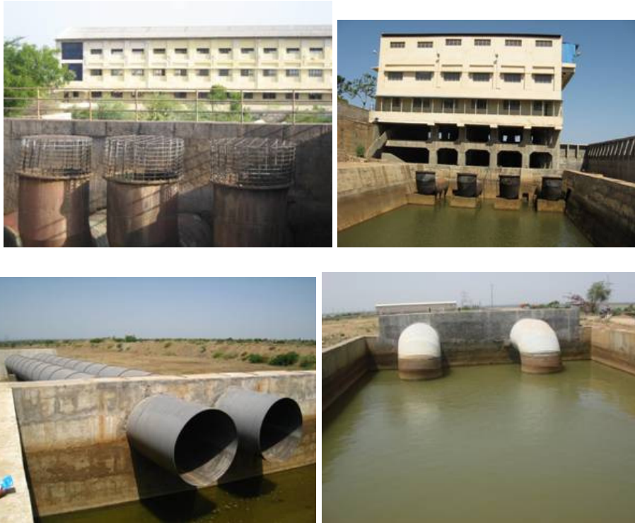
Plate 9. Diverse arrangements for outlet in delivery chamber: Vertical lift-up left in ALBC and right in ARBC – Horizontal in Mulwad and vertical siphoned in Mulwad.
