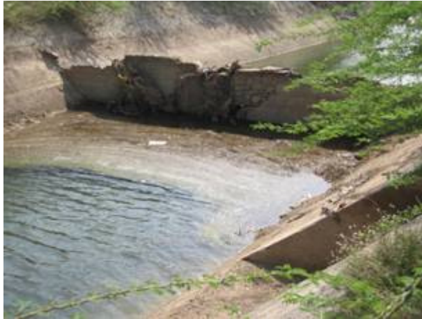
Plate 1. Temporary Cross-wall built for raising water level upstream ALBC at current low discharge [deteriorated and inefficient].
