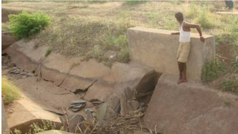
Plate 4. Slab and rocks placed at bed bottom to raise water head in Mulwad East Canal
