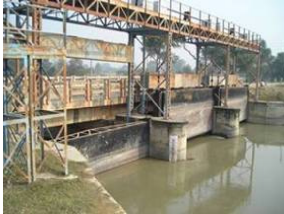
Plate 4. Typical Cross-regulator along the main canal (CR at 35.52 KM of JB Canal)
