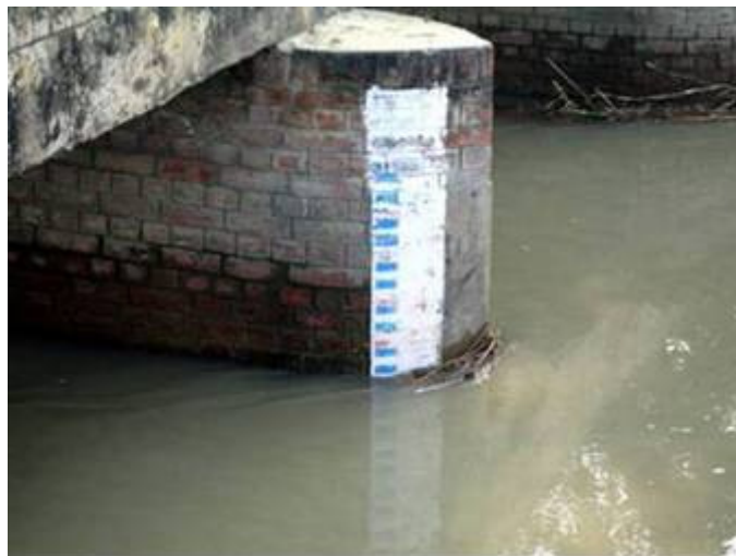
Plate 3. Gauge for discharge measurement on Jaunpur Branch canal
