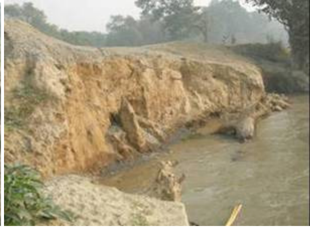
Plate 2. Jaunpur Branch Canal km.72 Slipping of canal side
