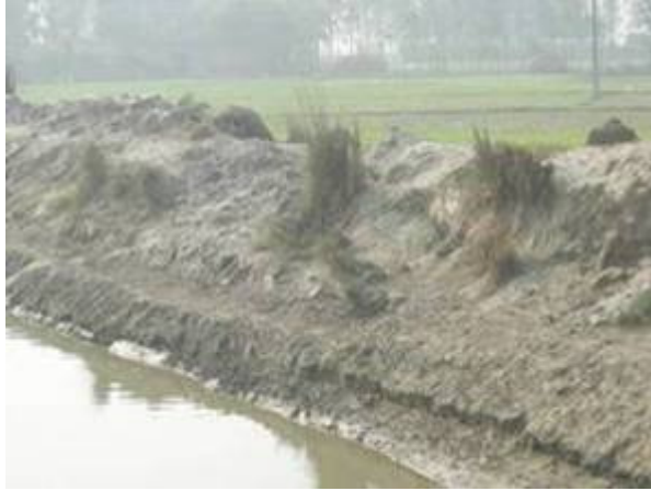
Plate 1. Jaunpur Branch Canal km.74 Heavy Siltation
