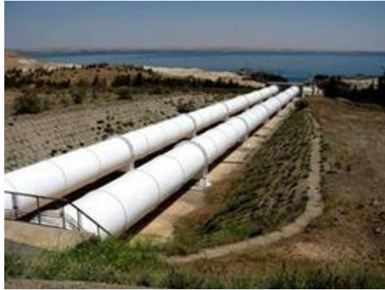
Plate 8. The lift raising pipes at Mounshaat-Al-Asad system (lake in the background)
