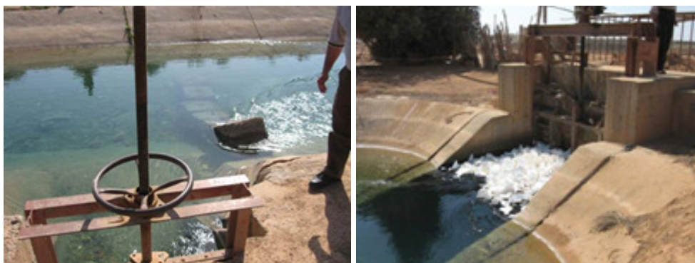
Plate 6: MC2 - C25 (left) Concrete blocks to raise water level at offtake while downstream X-Reg (right) is not used to control water level as it should be.
