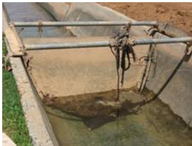
Plate 3: Portable gate along quaternary canal
