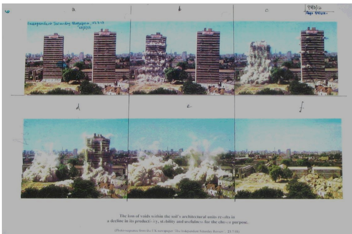
Figure 6: Controlled demolition of twin apartment-blocks. The interesting things happen in the spaces of soil architecture, as in a building. If the spaces are lost, the usefulness is lost, even though the physical parts remain.
